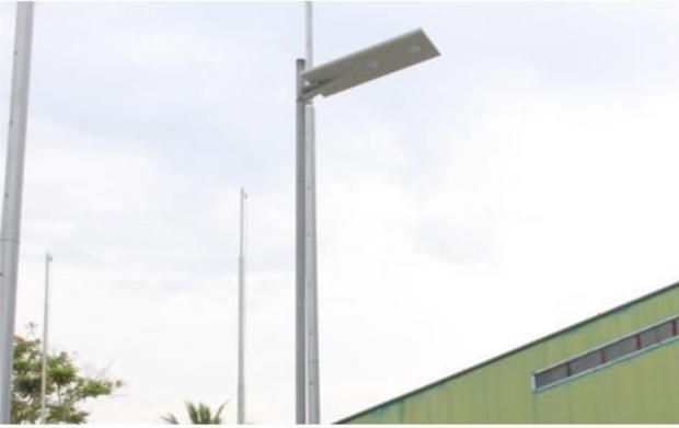
Title: Solar Street Lights Location: ACCESS External: 6 units
