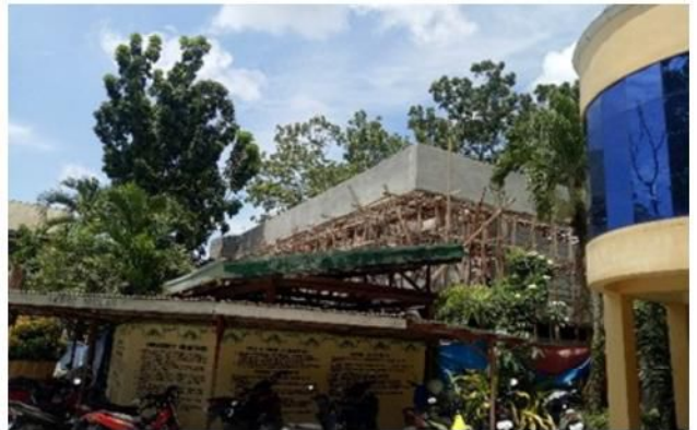
Title: Construction of Academic Building (Information Technology Building) Location: Isulan Campus ABC (Php): 7,500,000.00
