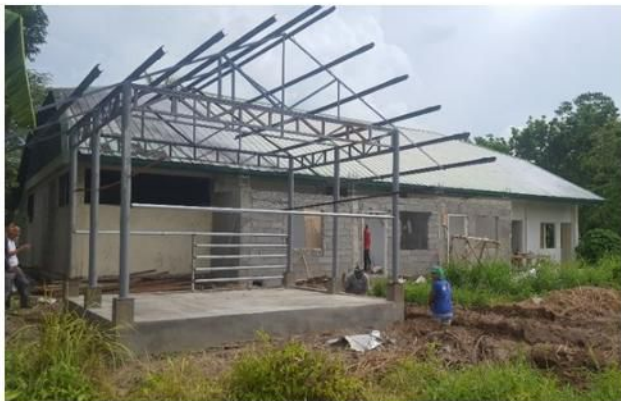
Title: Construction of Halal Slaughter House and Processing Center for Goat Location: Lutayan Campus ABC (Php): 7,500,000.00
